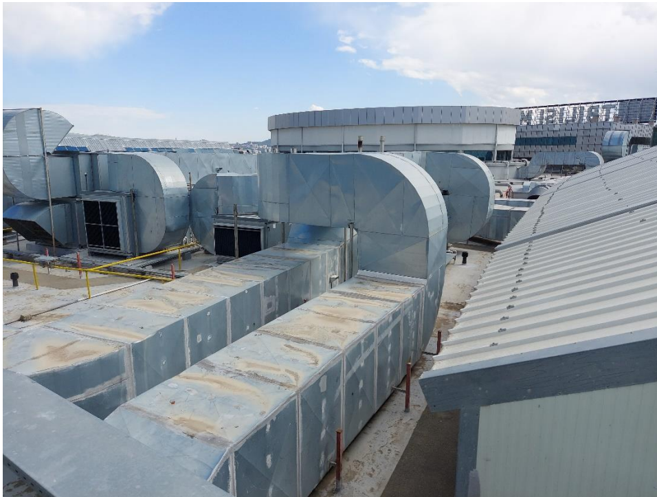
Typical air duct and equipment
